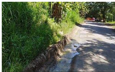
Figure 12. Puddles on the side of the road.
