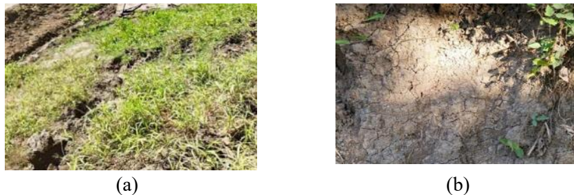
Figure 11. Cracking conditions on the ground at the research site (a) upper slope (b) lower slope.
